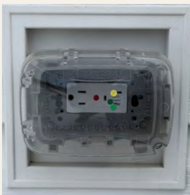
Exterior GFCI Receptacle
